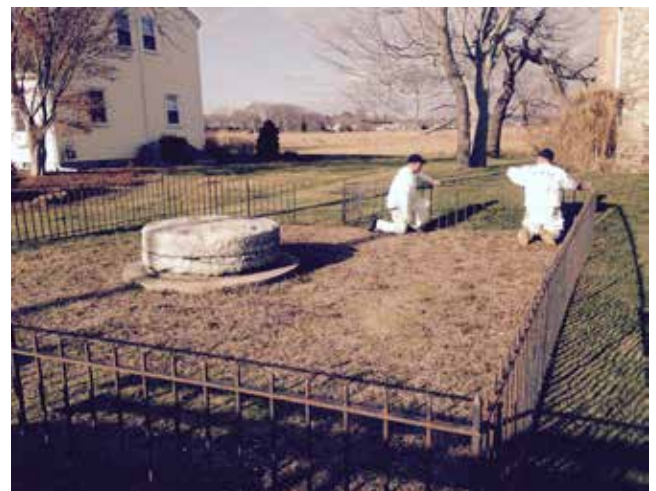
Painters work on the wrought-iron fence surrounding The Old Mill Stone, owned by the Historical Society. It had originally been part of the gristmill which operated at Saybrook Point. According to tradition the stone was brought from Holland in 1638. (Photo: Ed Armstrong)
