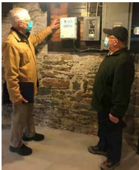
Old Saybrook Building Inspector (Tom Makowicki) and Ed Armstrong during the official electrical surge protection inspection.
